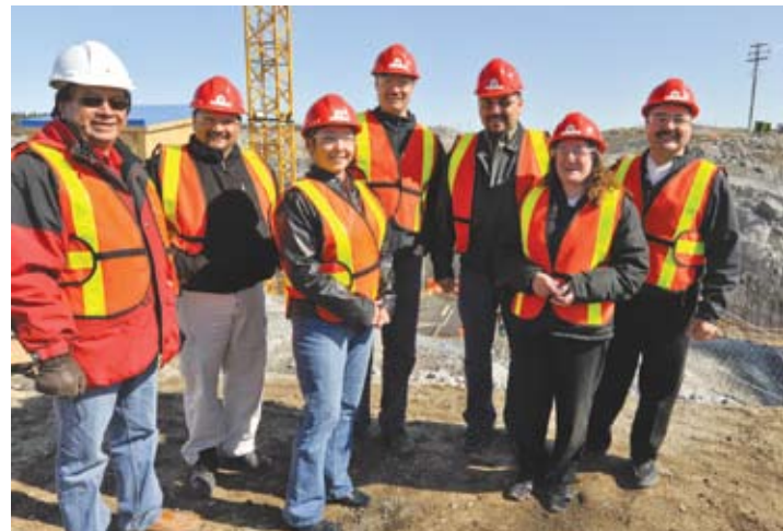
NCN Chief and Council on hand for the ceremonial commemoration of Wuskwatim's first concrete pour.
