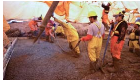
First concrete pour for Wuskwatim's above-ground structures. This phase of the project will provide good opportunities for general labour and skilled labourers.
