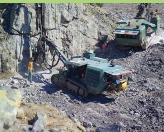
Top photo: main construction camp. Middle photo: rock stockpiling gravel for the finished grade of the access road. Bottom photo: drilling machines at work on Phase 2 rock excavation for the principal structures and channels.
